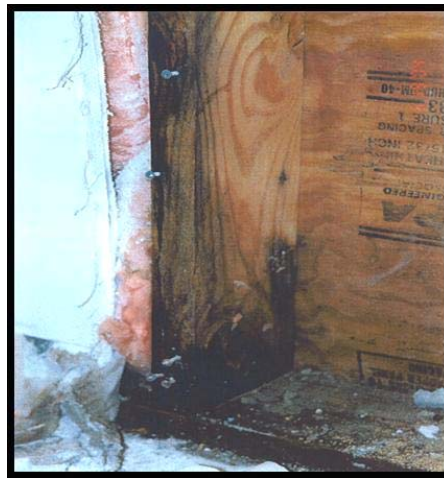
Figure 8. Water staining of framing members.
