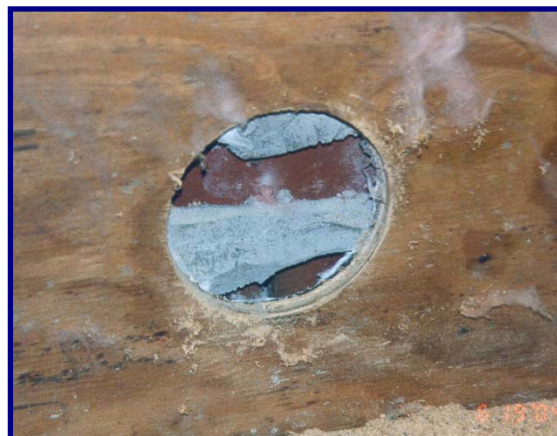
Figure 9. The band of mortar running horizontally would obstruct downward migration of moisture to the flashing and not be expelled to the exterior.
