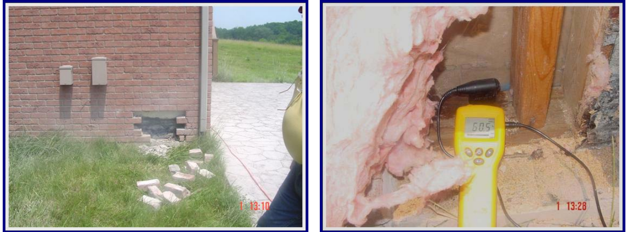
Figure 4. Intrusive inspection of the wall cavity at the south side of the north elevation; see corresponding thermogram in Figure 2. Elevated moisture levels were measured in the building materials. Fiberglass batt insulation was colonized by fungi (18,680 CFU/g) and was dominated by Aspergillus versicolor (91%).
