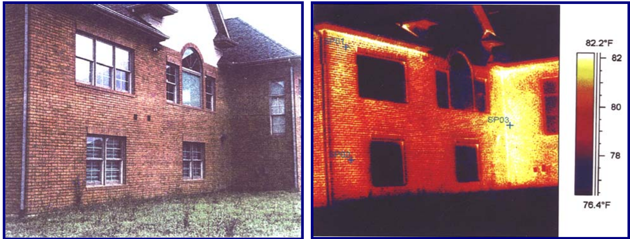
Figure 2. This thermographic image taken at the south side of the north elevation on June 25 showed thermal anomalies in the brick veneer. The suspected wet areas are relatively warm and clearly visible in this thermogram as white and yellow areas. Cooler, dry areas are red, purple, and black. The color bar shows the measured temperature range of 76.4 to 82.2 °F. The ambient temperature was 76 °F and the object distance was 50 ft. See Figure 4 for observations made during the intrusive inspection of the wall cavity.
