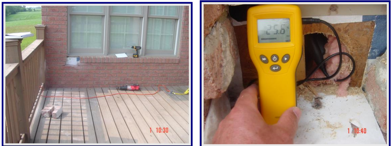
Figure 5. Intrusive inspection of the wall cavity at the south end of the north elevation; see corresponding thermogram in Figure 3. Elevated moisture levels were measured in the building materials. Fiberglass batt insulation was colonized by fungi ( 9.71E+05 CFU/g) and was dominated by Acremonium strictum (76%) and Aspergillus versicolor (22%).
